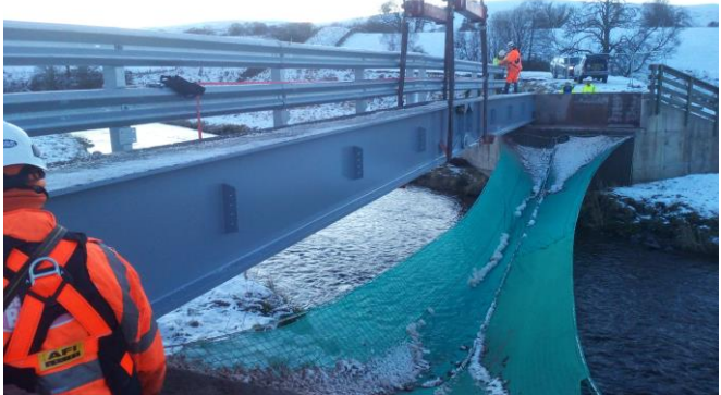
Minnygap Wind Farm, Moffat
